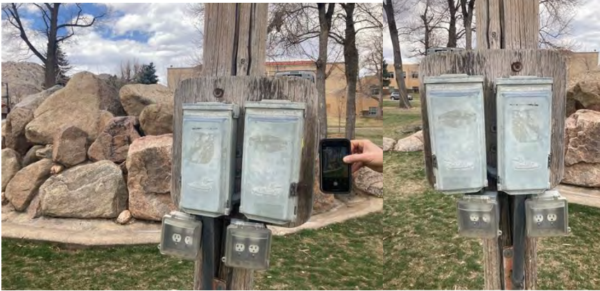
Location #11: Electrical Boxes near Cameron’s monument
