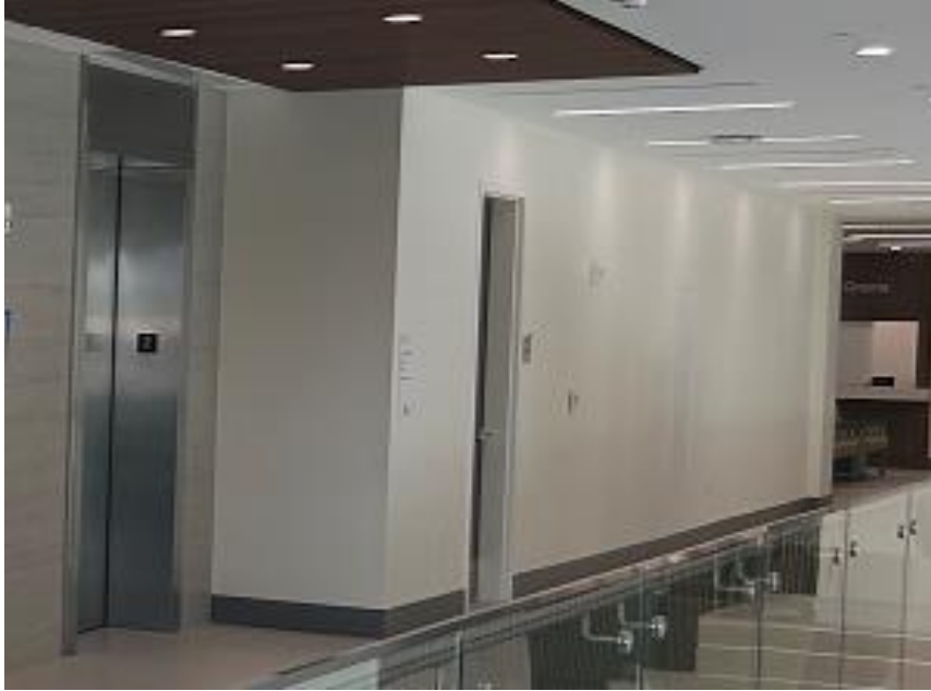
(Qnt. 2 - Wall Size 18.0ft W x 8.11ft H – Hallway to the right of the elevator but also visible from 1 st floor)
